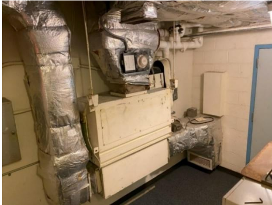
Figure I-7 Antiquated Boiler with Suspected Asbestos in Foil Duct Insulation
